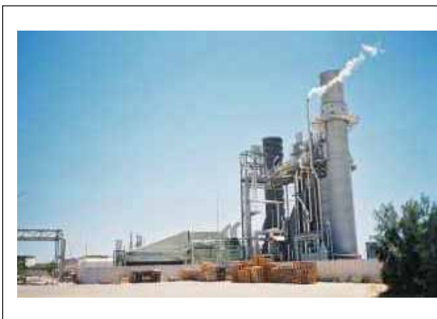
Combined cycle co-generation site
